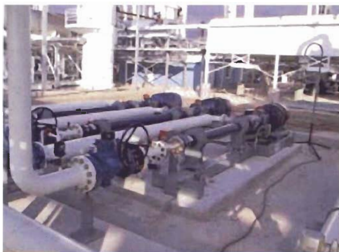
FIG. 7 REDA pump installation at the Bishop facility.
