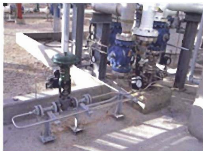
FIG. 8 Control valve and thrust bearing filtration system.
